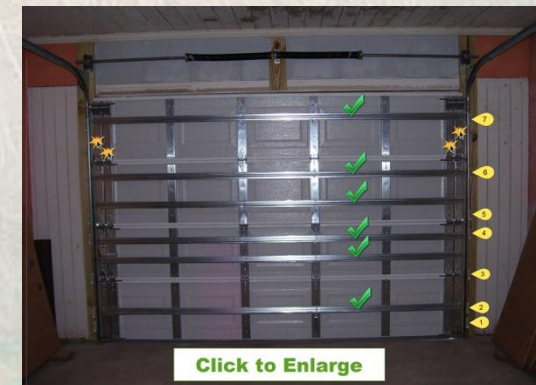
Wind-rated garage doors 7 braces
