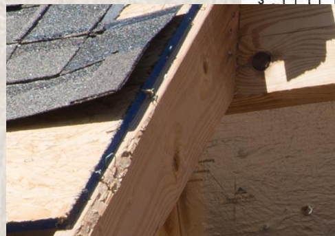
Stapled roof deck Missing deck nails
